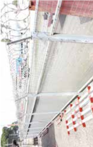
358 High Security Fencing with razor wire and barbed wire.
